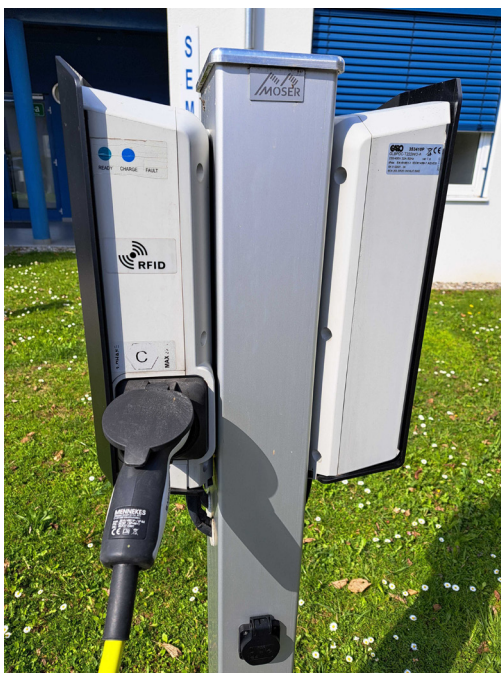
Fig. 5: Charging Pile Connection
